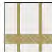
Check Windowpane Putty
